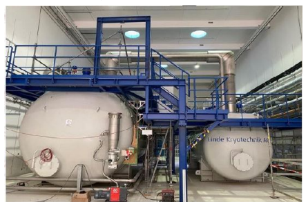
Cryo Plant and cooling water system
