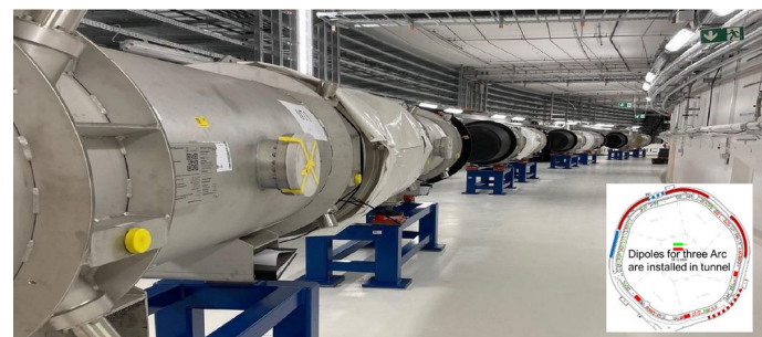
SIS100 accelerator tunnel
